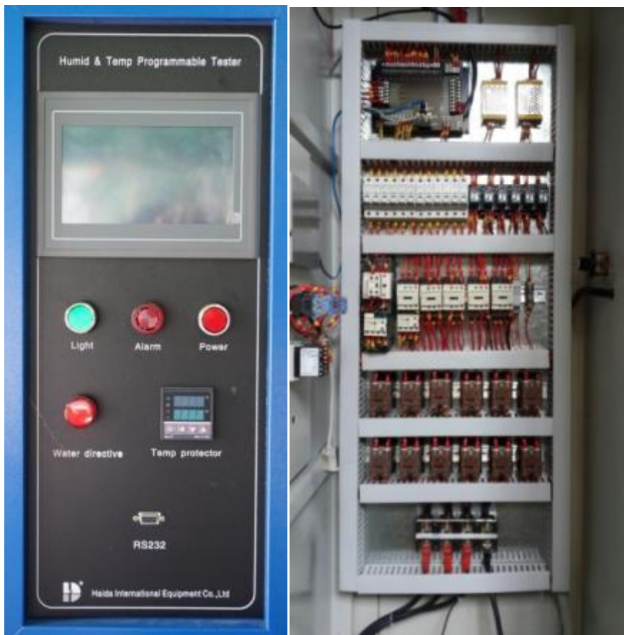
CONTROL PANELCIRCUIT BOARD
